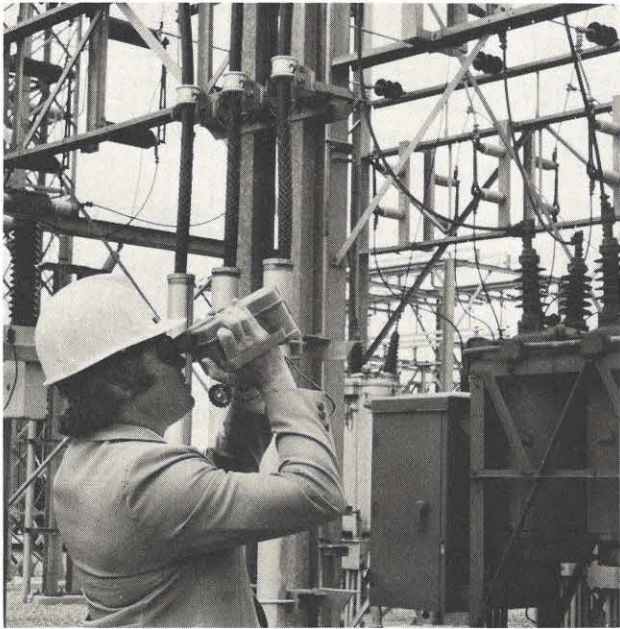
Jay Johnson uses the Probeye to check for hot spots in bus work connections at Cloverdale Station.
