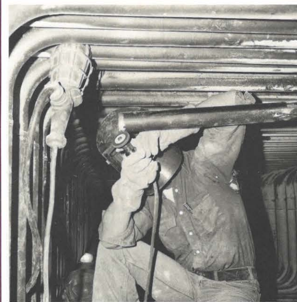
D. W. Dye, maintenance mechanic, and a certified welder in the Amos Unit 2 reheat section repairing tube platen for weld.
