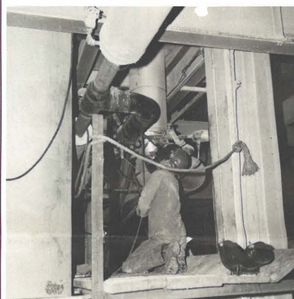
T. M. Henry, maintenance mechanic, repairs damaged section in 6-inch steam header to slag blower.
