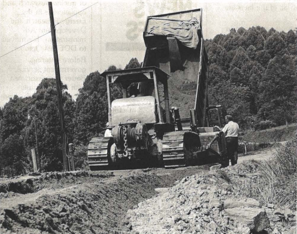
Cement-treated bottom ash from John Amos Plant is being spread on a secondary road in Kanawha County, West Virginia.
