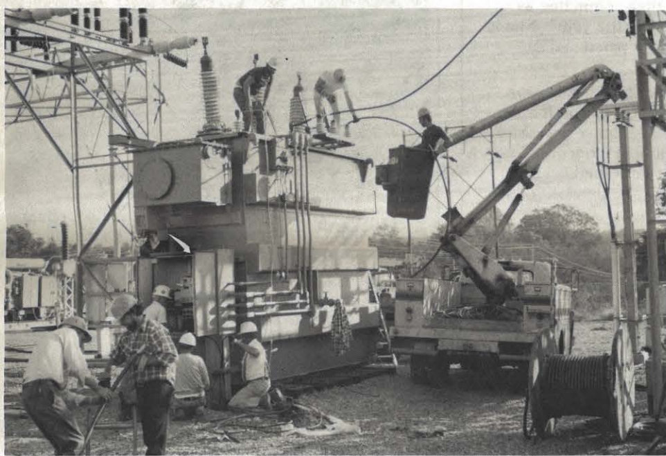
Lynchburg station employees install a new 20 mva 138/12 transformer at the Forest Station. The old transformer was damaged by lightning when a severe electrical storm hit the area on August 9 and interrupted service to over 3,300 customers. The distribution at Forest Station was switched to other sources, and a mobile transformer was brought in from Roanoke and placed into service the following day.
