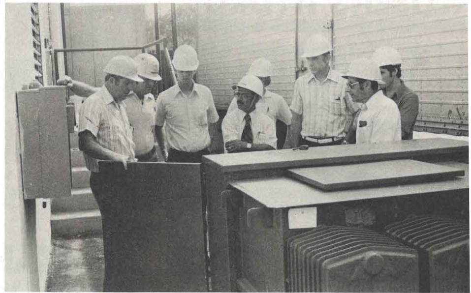
Observing the installation of underground service and transformer at a new Winn-Dixie store in Lynchburg are, l. to r., Tom Witt, Kenneth Triplett, Tom McConaghy, A. C. Channaiah, Dave McFaden, Norman Fowler, Jim Dorman and Doug Fitchett.
