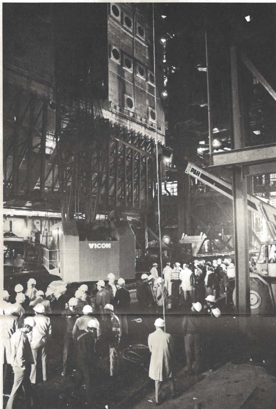
Coal company executives view the massive boiler at Mountaineer plant before the B&W unit was totally enclosed.
