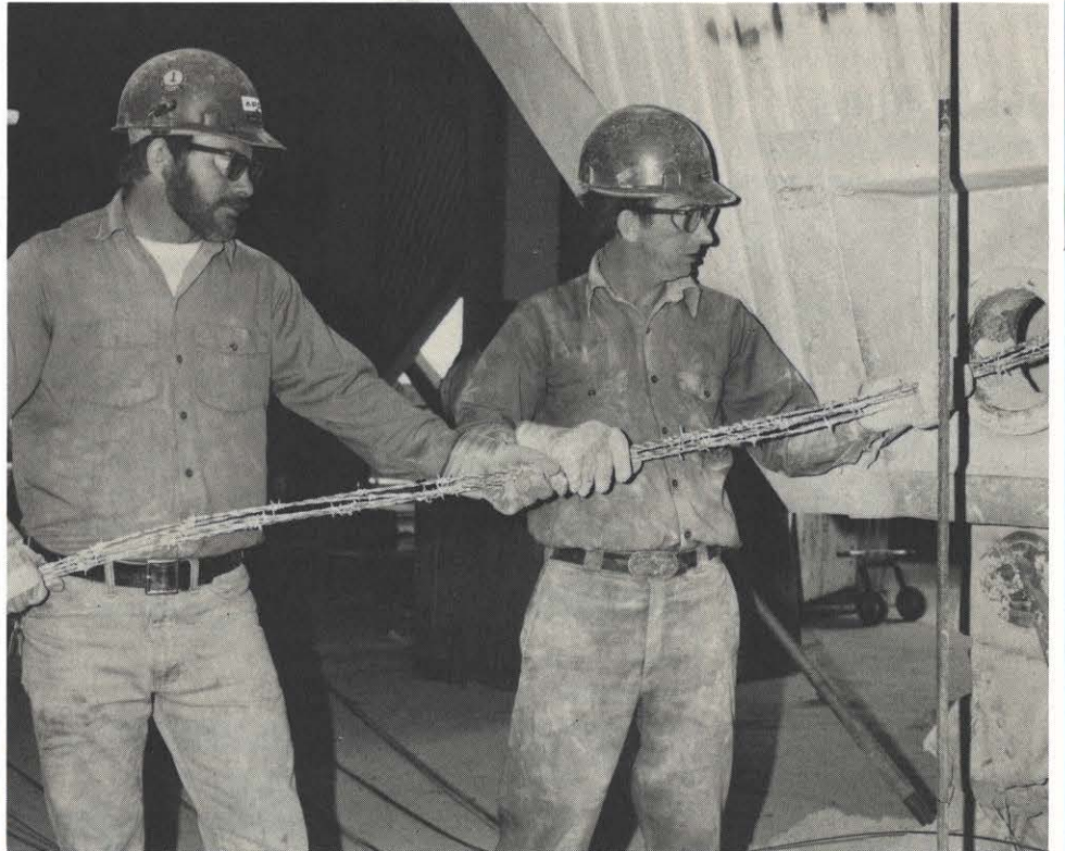
S. W. Cover, left, and J. T. Pickering, both maintenance mechanics B, pull wire from the hopper hole.
