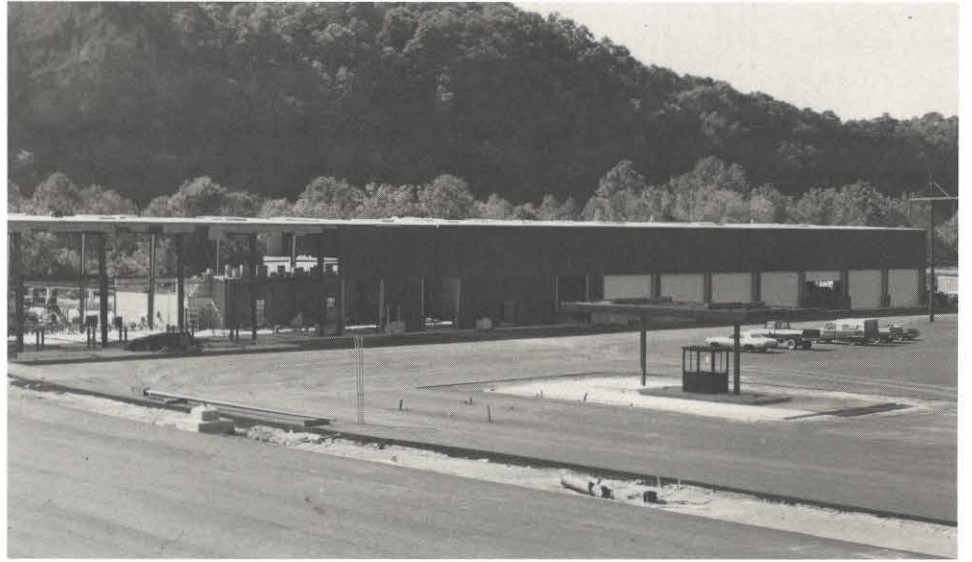
Work on a new $2.3 million service building for Kingsport Power Company has passed the halfway point. The building structure and outside paving have been finished and inside work is underway. The 40,000 square foot metal and brick building is scheduled for completion in May 1981. C. A. Davidson is resident engineer for the project.
