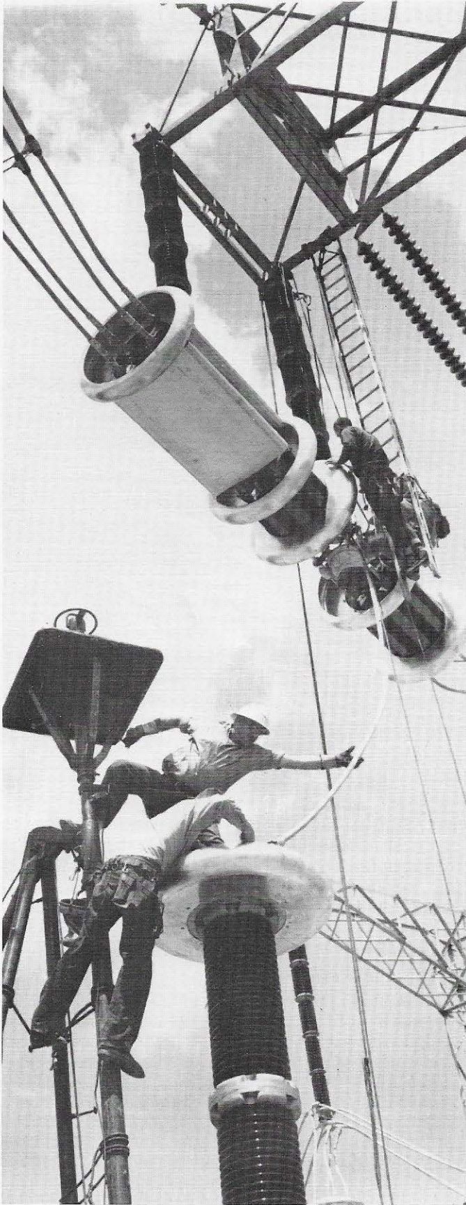
And at the Apple Grove (W.Va.) test line, more AEP research in 1961-68 led to the world's first 765,000-volt transmission lines.
