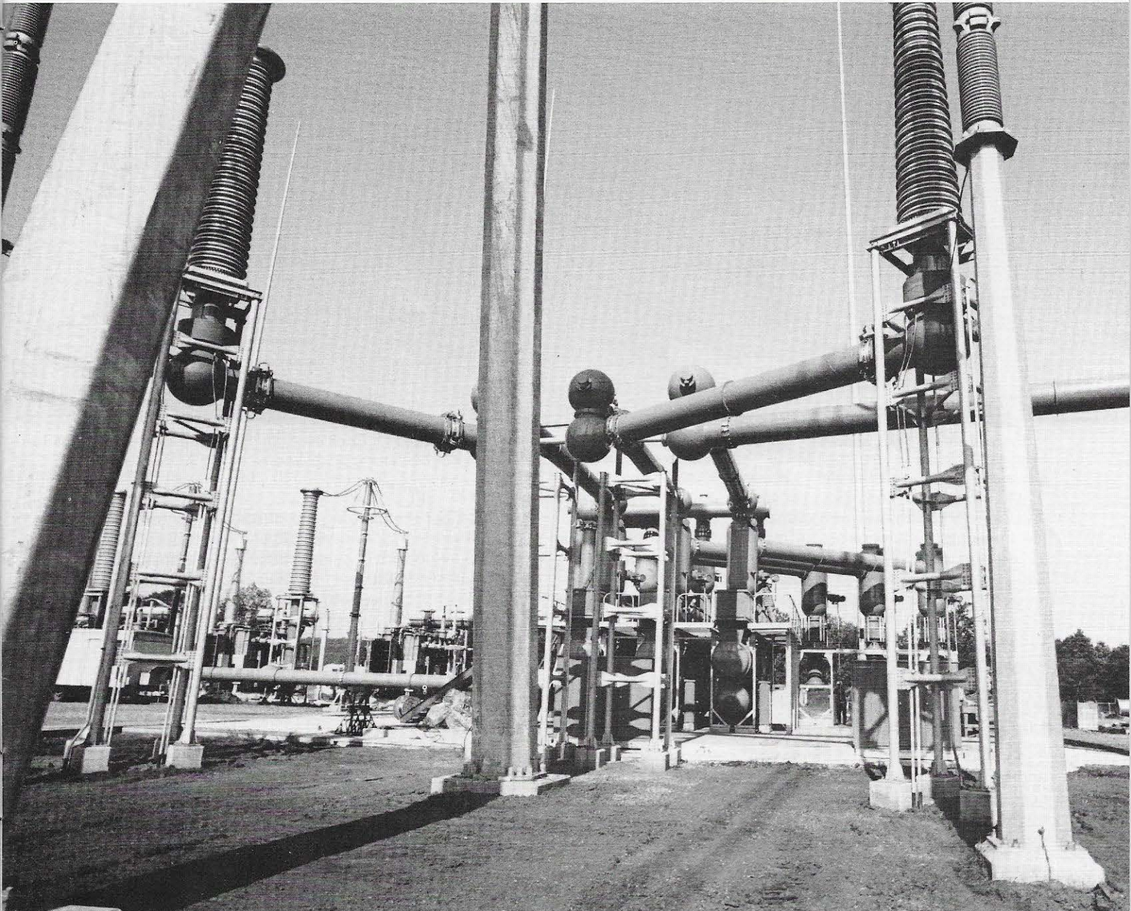
Appalachian Power Company's Joshua Falls transmission station near Lynchburg, Virginia, was the scene of the world's first use of a gas (sulfurhexafluoride, SF 6 ) to replace air as insulation in a 765,000-volt facility, enabling a sizable reduction in station size and land requirements. Earlier applications of SF 6 had been made at lower-voltage stations belonging to Indiana & Michigan Electric Company in Fort Wayne and South Bend, Indiana.
