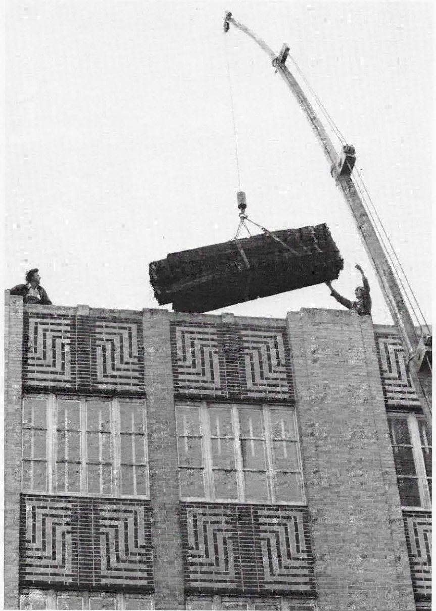
The first load of the outdoor coils is being hoisted from the roof of the headquarters building by a 100-foot crane.
