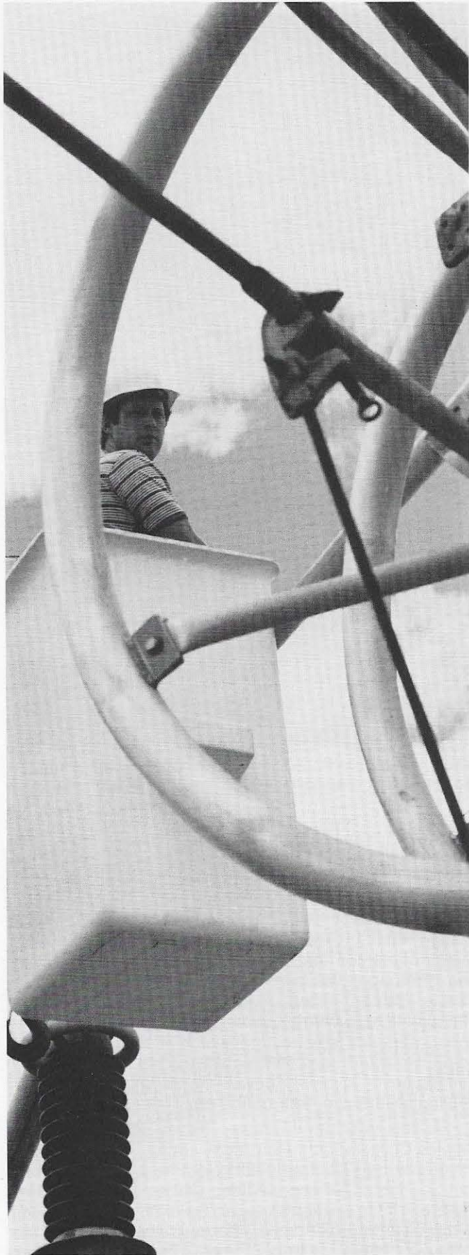
Special studies involving the 765,000-volt-line phenomena are performed at the lab. Here, John McCallin, senior technician, changes the test line arrangement.
