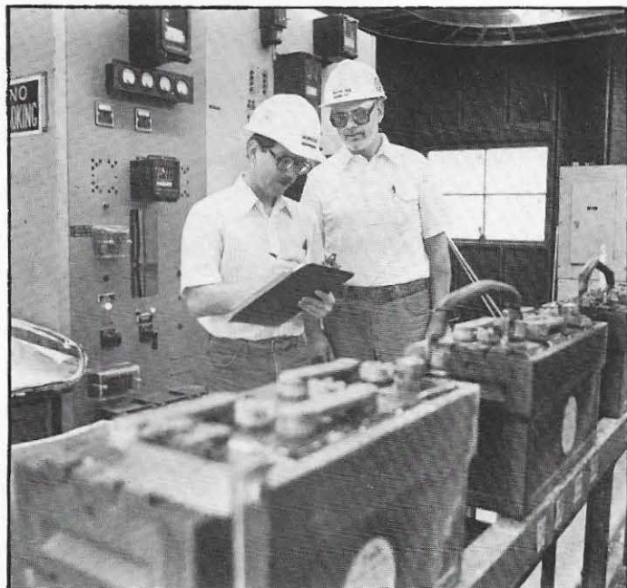
A substation control building's condition and safety environment is rated by safety audit committee members Bob Heil and Jim Reid.
