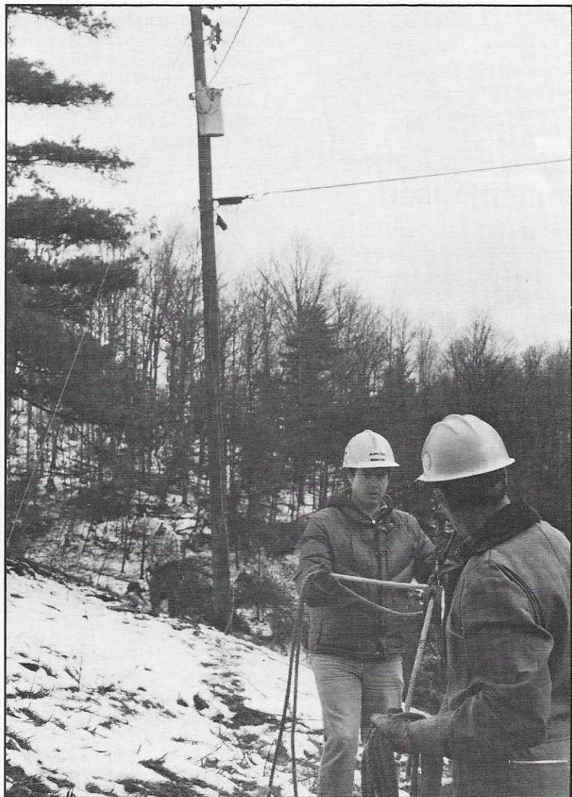
An Abingdon division line crew restores electric service following the mid-December snow storm. Many of the trouble calls were in isolated areas.
