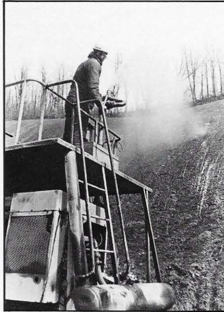
At Cedar Coal Company and Southern Appalachian Coal Company, hydroseeding crews spray a slurry of grass seed, fertilizer and water on regraded land after surface mining.
