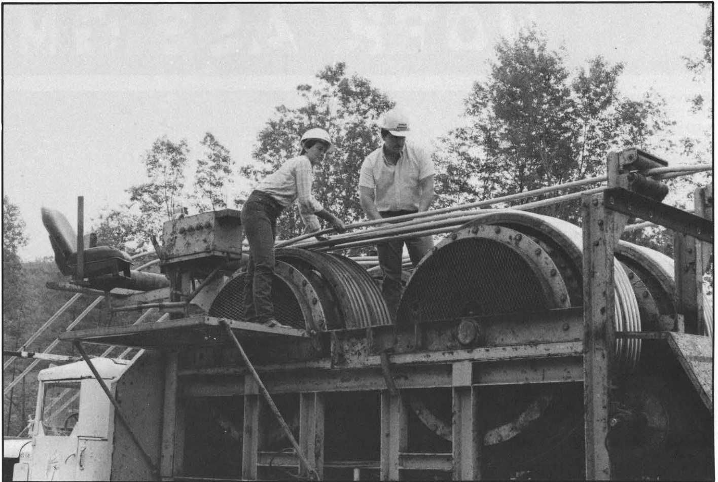
Dianna Curtis, left, and Jack Gardner check the conductor for damage or loose stranding and for correct threading through the tensioner.
