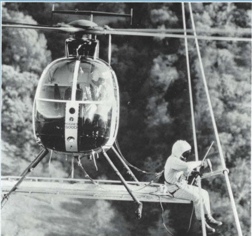
In this publicity photo from Haverfield, a repairman works on an energized 500 kv line.
