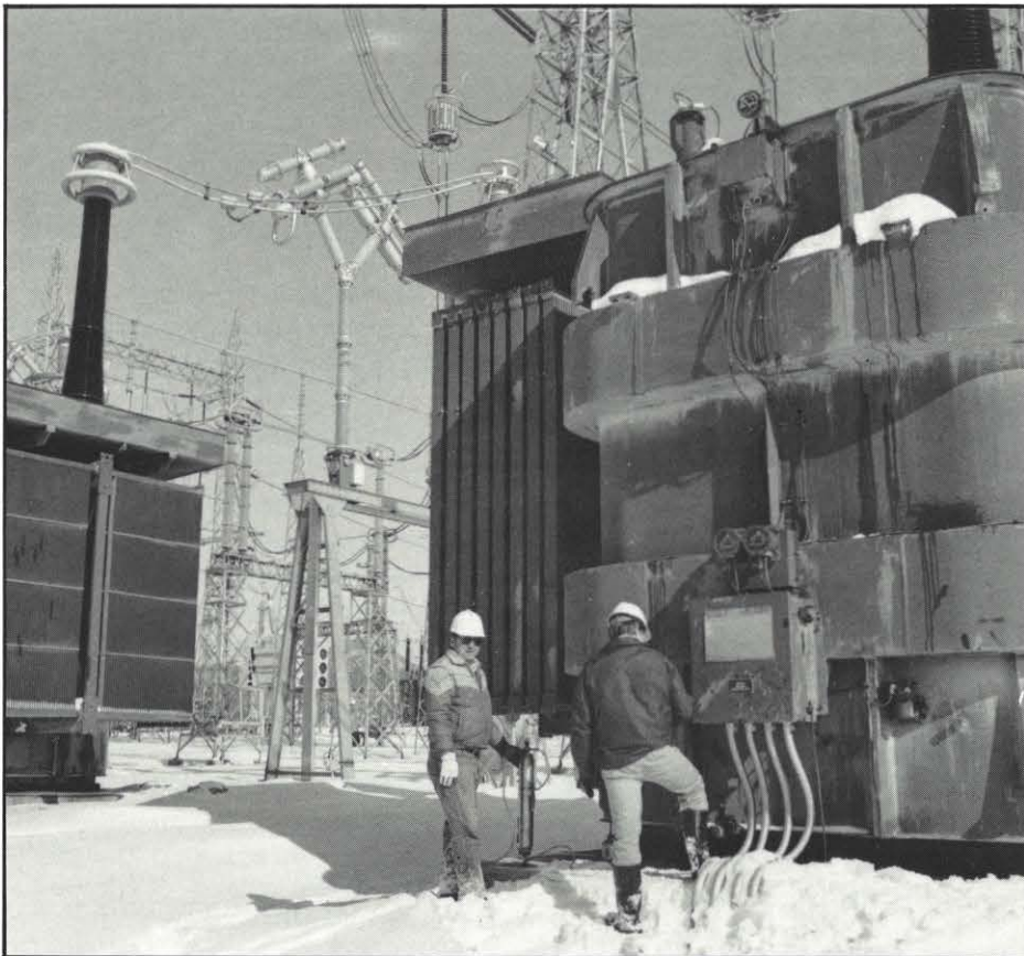
Roy Painter, transmission station mechanic A, left, and Joe Coley, electrical engineer, both of GO T&D Station, work in the Cloverdale Station near Roanoke.
