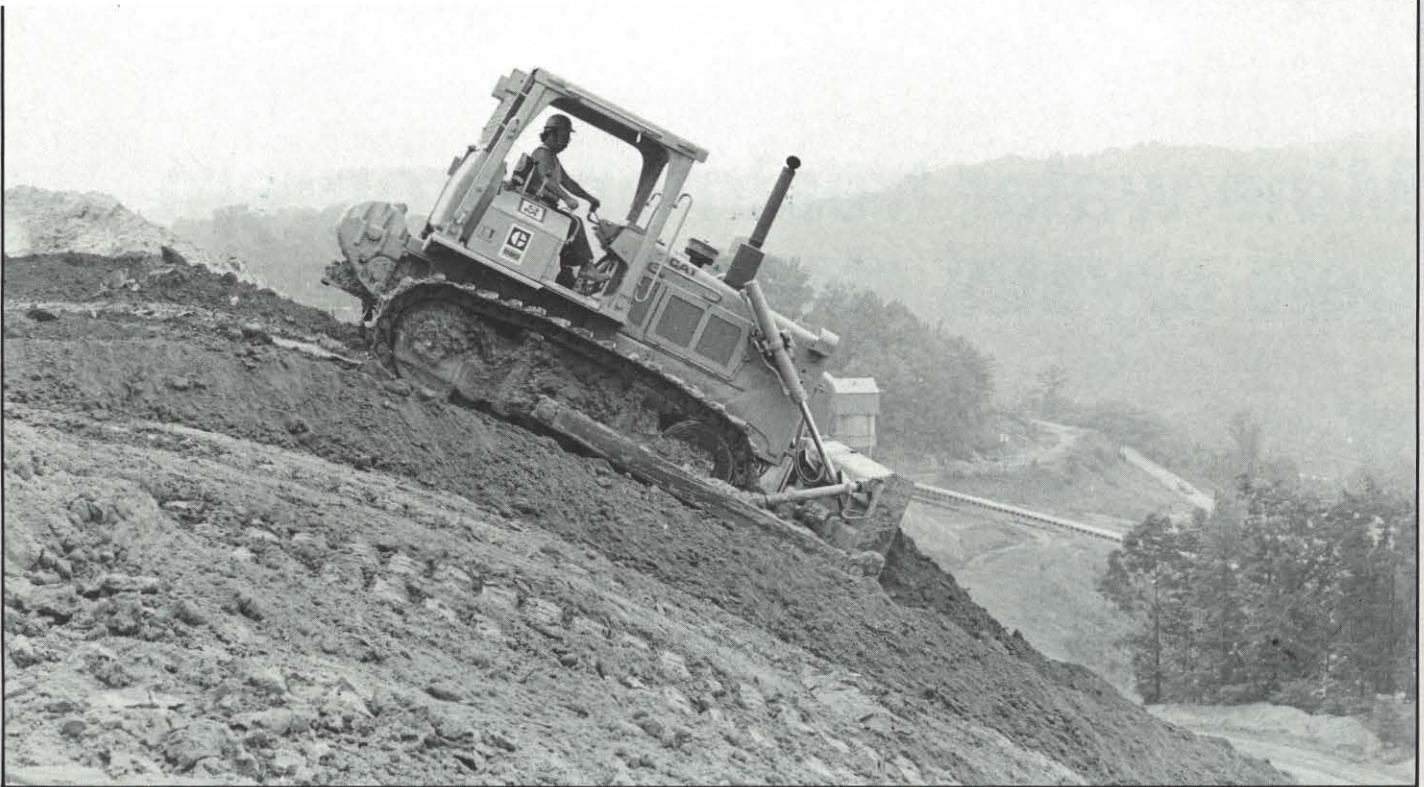
Once a refuse area has reached the end of its "life" at an AEP coal-mining operation, it is reclaimed and returned to its natural, productive state. At Martinka's Powell refuse area, a bulldozer operator grades an area prior to seeding.
