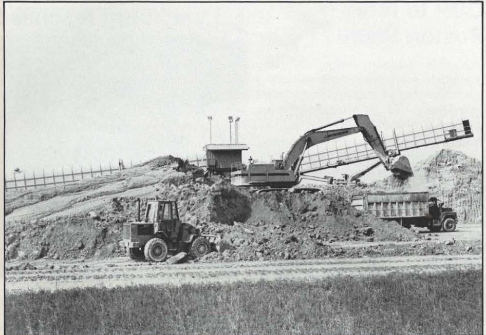
Sludge from the Conesville scrubbers is loaded onto trucks for transport to the nearby on-site landfill. Behind the shovel is the conveyor system that carries the processed waste material from the sludge treatment facility.
