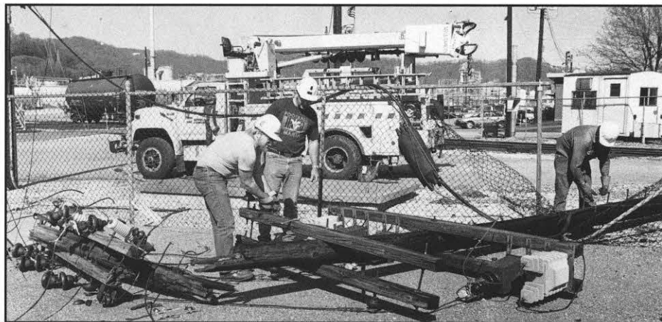
Appalachian Power crews, contractor crews, and crews from other AEP operating companies were out around the clock repairing storm damage. L. to r., Greg Hanshaw, Charleston line mechanic B; Jim Hicks, line mechanic A; and Kenneth Looney, line mechanic C, replace a utility pole at the Occidental Chemical plant in Belle, WV. Photo by Chet Hawes, Charleston Daily Mail.
