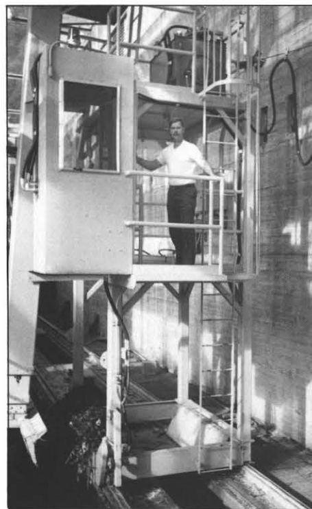
Jim Stamper, hydro mechanic B, prepares to operate the new trash rake at London Hydro Plant. Its new telescoping hydraulic-arm design offers many advantages over the old cable-operated design
