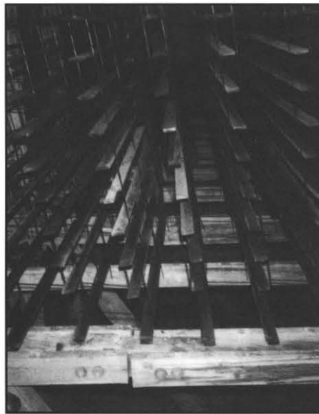
During the period from Fall 1987 to Spring 1990, approximately 60 percent of the tower structures and 100 percent of the tower fill were replaced on Clinch River Plant cooling towers 1-5. The refurbishing should lengthen each tower's life by approximately 20 years. This photo shows the new fill.
