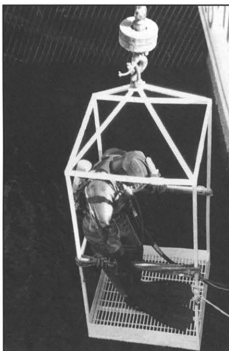
One of the International Underwater Contractors divers descends into the waters of Smith Mountain Lake.
