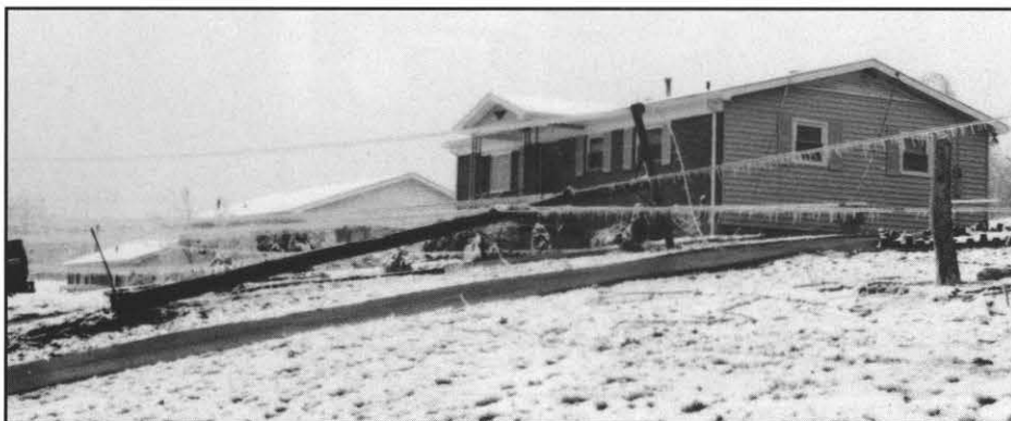
A broken utility pole and downed lines narrowly missed this customer's house.
