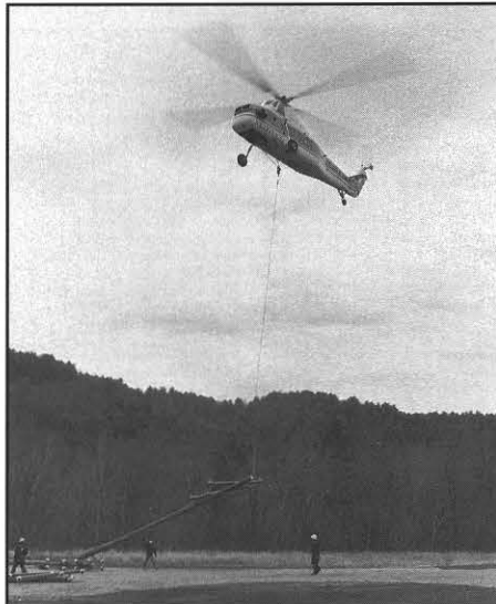
Carson Helicopter of Perkasie, Pa., was used to set 35 replacement poles in the Byllesby-Buck-Ivanhoe 13.2 kV line in Carroll County, Virginia.
