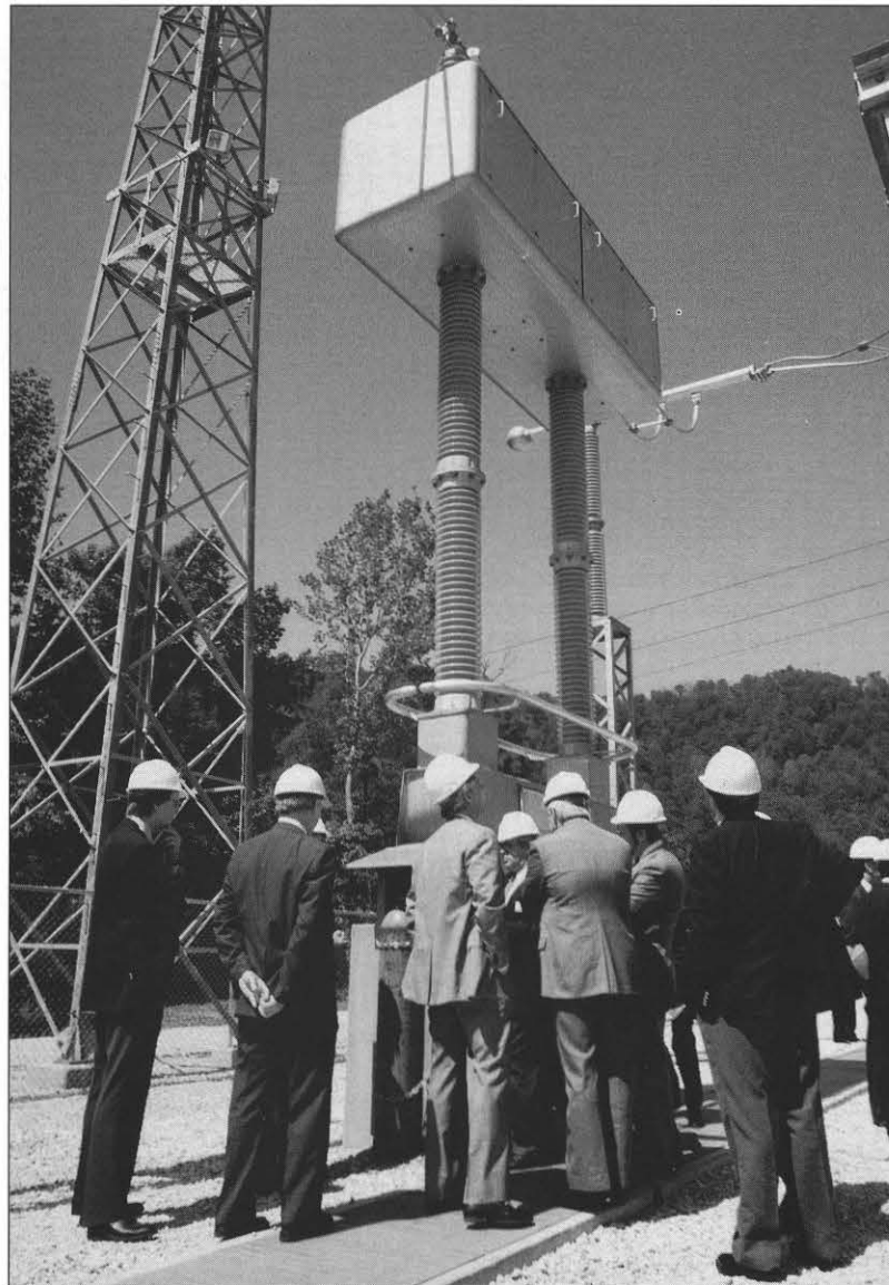
Charleston area civic leaders along with officials of American Electric Power, Appalachian Power, and ABB Power Systems inspect the world's first outdoor thyristor control switch installed in the Kanawha River Plant switchyard.
