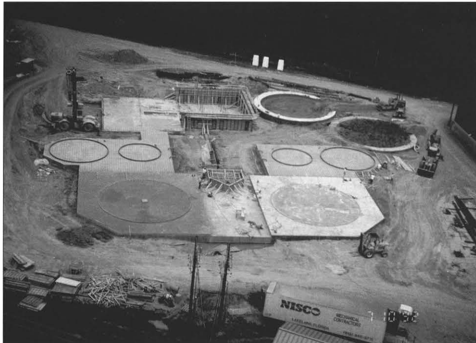
Clinch River's new wastewater treatment facility is being constructed on a 2.1-acre site between cooling towers No. 3 and No. 4.
