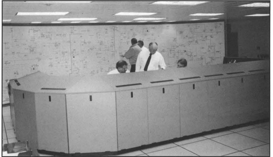
This view of the Abingdon Regional Dispatching Center shows the new mapboard and desk console housing radios, telephones, and computer CRTs.
