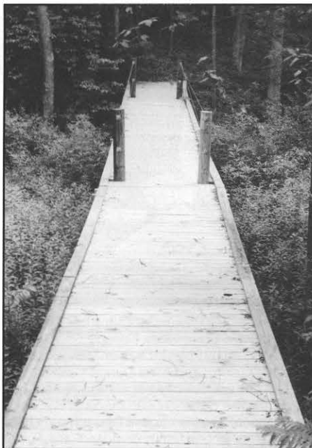
The Beckley Line Department constructed this footbridge across a wet area along the trail.
