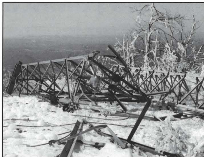
Tower 264 on the 345 kV transmission line collapsed February 11 during the worst ice storm ever to hit Appalachian Power's service area.
