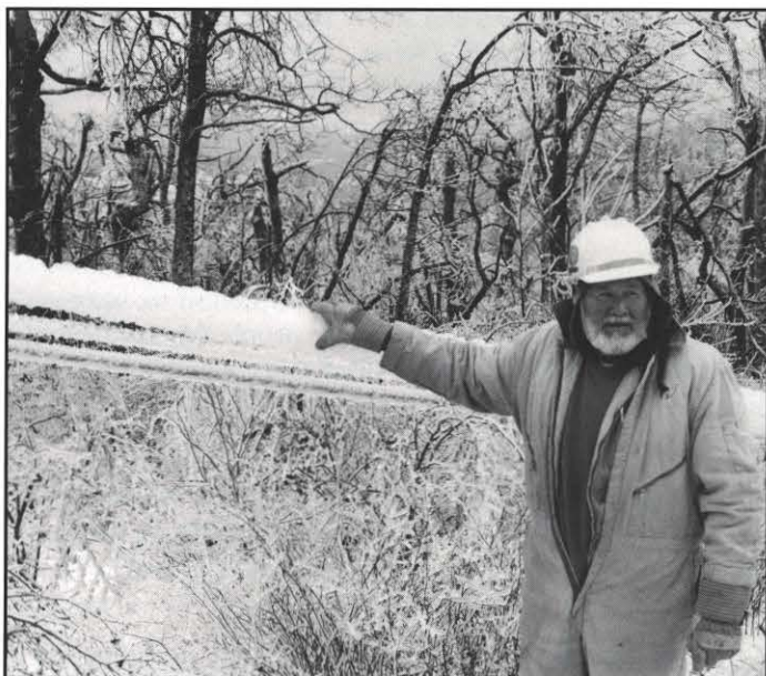
George Goodall, Jr., transmission line crew supervisor, GO T&D Transmission, Turner, holds his hand on the downed tower's static wire, which had 6 to 8 inches of ice accumulation. The conductors underneath, through which electricity flowed, had lesser amounts.
