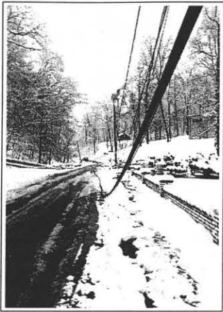
According to APCO officials, about 36% of it's 441,000 Virginia customers were without power during the February 11th storm.
