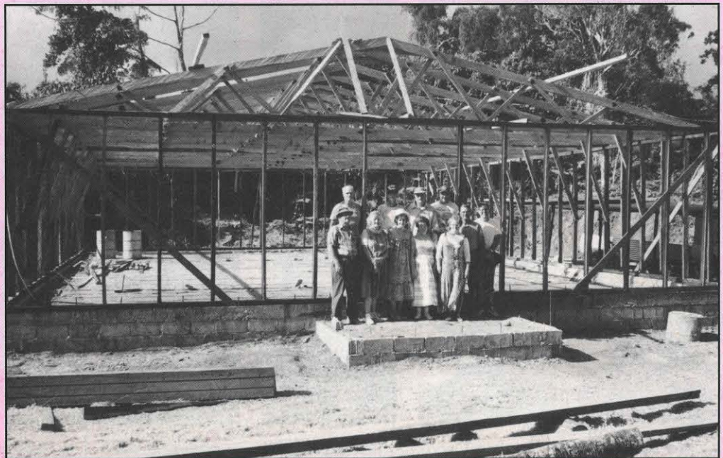
The missionary group from the Cross Lanes Bible Church pose at the entrance to the church building under way in the village of Nabua.
