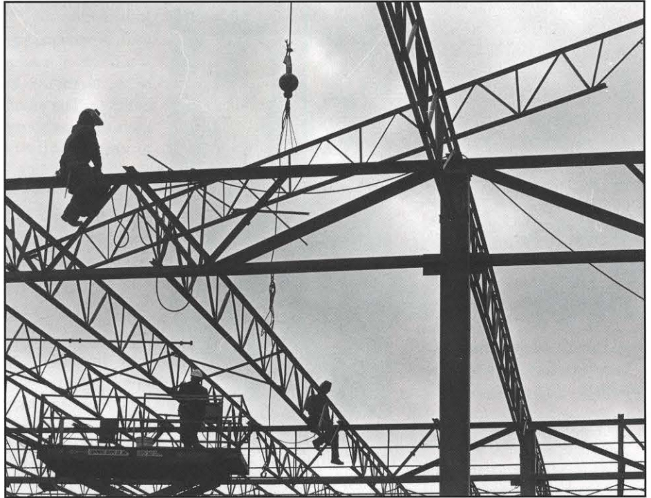
The Magnolia Mills building under construction in Appalachian Power's Carroll County, Va., service area is beginning to take shape. The building is expected to be completed in May. Photo courtesy Larry Chambers, Galaz Gazette.
